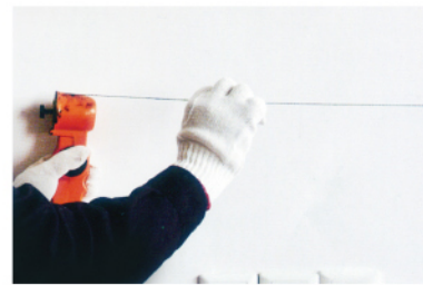
◆ 根據施工圖紙彈墨線 Lightly mark wall to indicate level hanging position.
